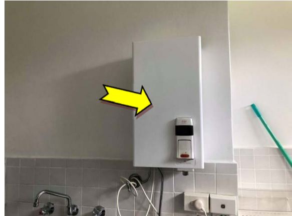
Photo 2. Interior, kitchen, hot water heater – suspected SMF internal insulation material.
