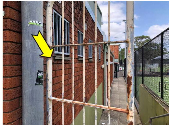
Photo 4. Exterior, throughout, fences – lead-containing white upper coloured paint system.
