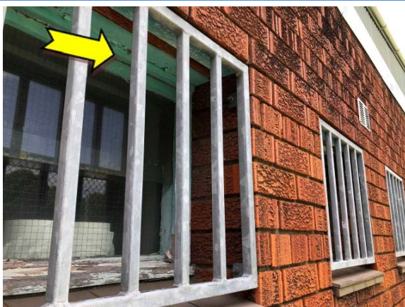
Photo 5. Exterior, throughout, window frames – lead-containing blue upper coloured paint systems.
