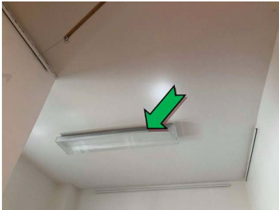
Photo 3. Interior, adjacent entry, double tubed fluorescent light fitting – suspected non PCB-containing capacitors.
