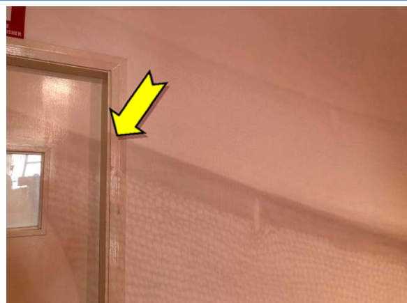
Photo 6. Interior, throughout, windows and door frames – lead-containing beige upper coloured paint system.
